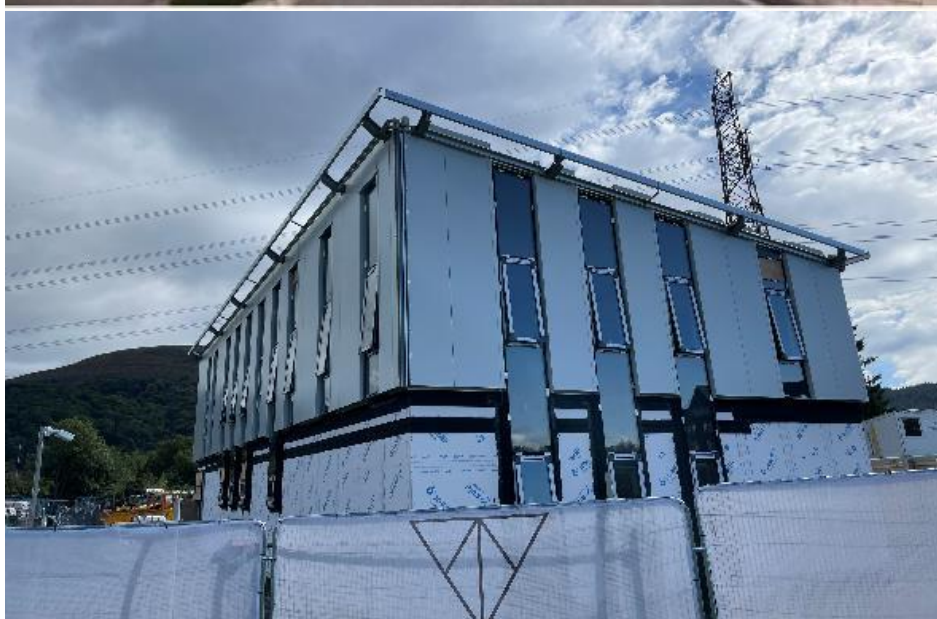
Artist impression of new police station located near A465 at Llanfoist (above) and now under construction (below)
