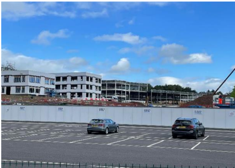
Abergavenny King Henry VIII School – image of the new approved school (above) and the development now under construction (below)
